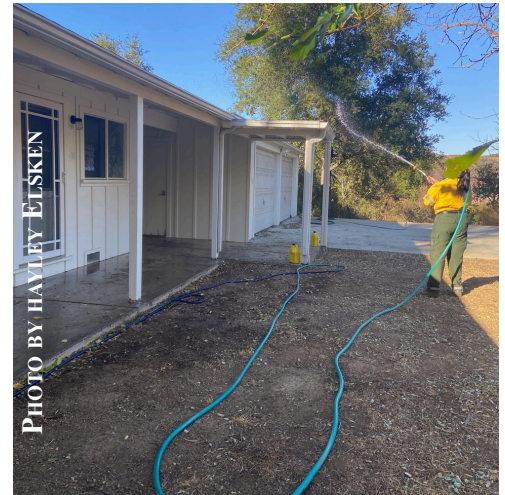
Angeles District employee rewetting gel on state park building during the Palisades Fire.
