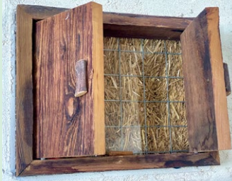
A pair of small cupboard doors set in a BARC wall reveals the straw bale infill.
